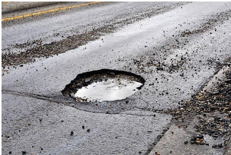
Figure 2 Road Damage Image
