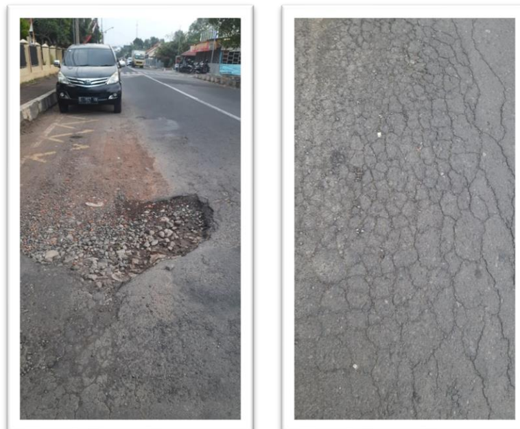
Figure 3. Photo of Road Damage Types on Jalan Laswi
