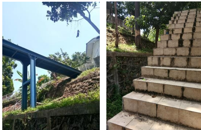
Figure 3. Lack of handrails on the stairs
