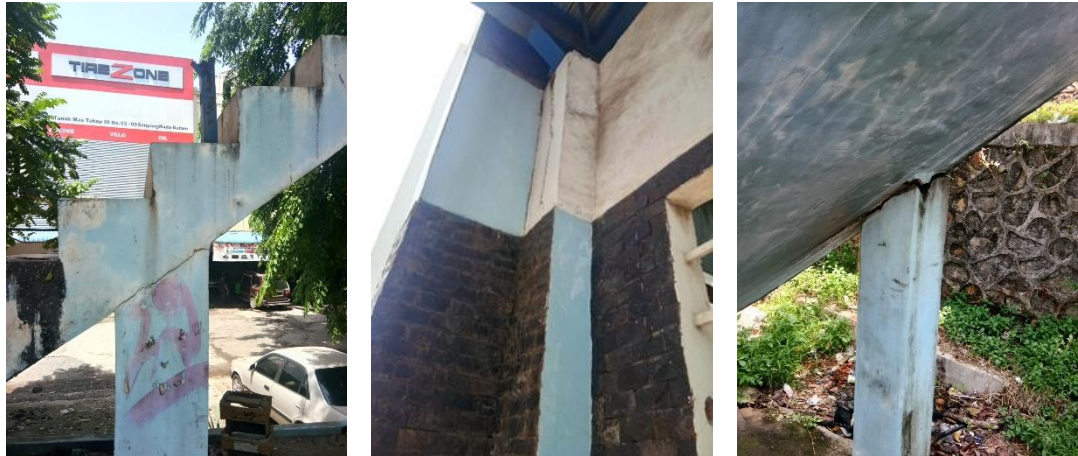
Figure 2. Deterioration of pedestrian bridge the first stair column
