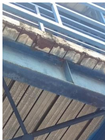
Figure 4. Corrosion on the steel deck
