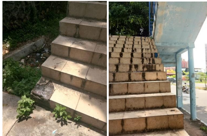
Figure 5. Weeds growing on the staircase
