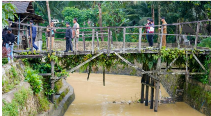
Figure 2. The Condition of the Kanaan Bridge Before the Reconstruction (Source: Google, 2023)
