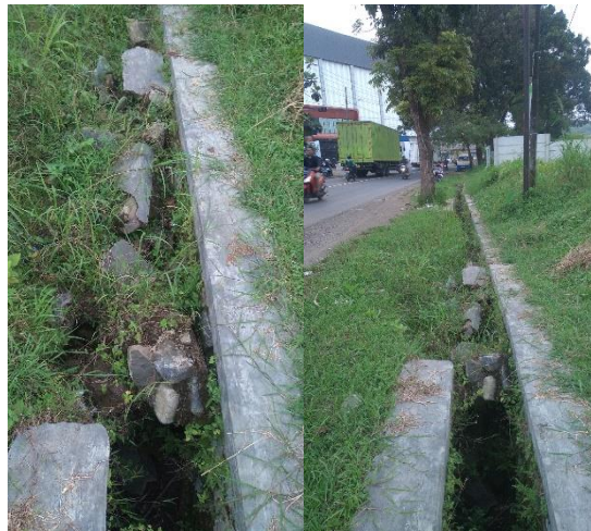
Picture 1.9 STA 2 + 951, with a collapsed drainage wall.
