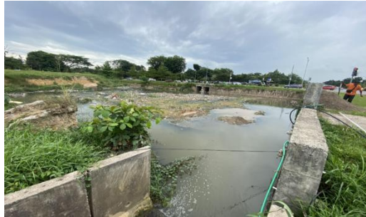
Figure 2. Existing Drainage Conditions in Batam Centre Sub – District
