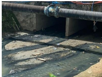
Figure 9. Sediment build after storm water receded, Nagoya Sub – District, Source : Real time observation
