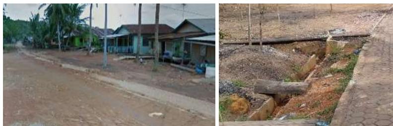
Figure 5. Drainage System that was not Visible in 2016 (Left) and Partially Constructed in 2021 (Right)
