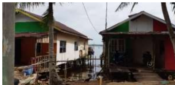
Figure 8. Building Materials whose Visual Quality is Maintained (Painting is Done), But There Are Still Defects in Parts that are not Maintained
