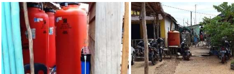
Figure 4. Clean Water Reservoirs in Kopak Jaya 007 Restaurant (Left) and in One of the Residential Buildings (Right)
